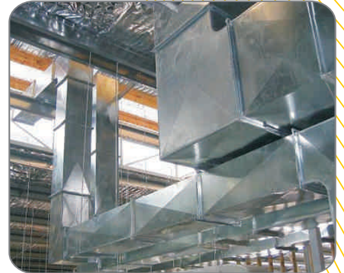
GI SQUARE DUCTWORK
