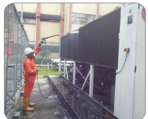
AIR COOLED CHILLER CLEANING
