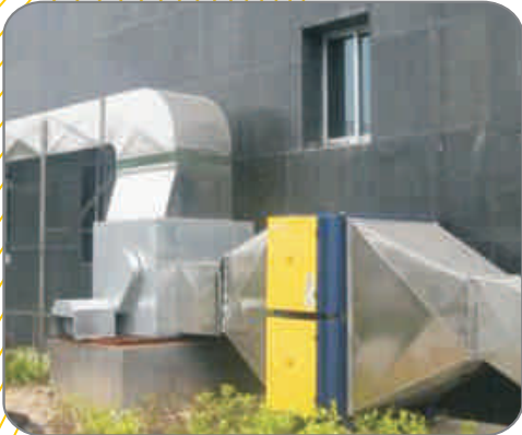
KITCHEN EXHAUST COMPLETE SYSTEM
